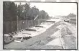
LANDSLIP REPAIR FILLS 6
