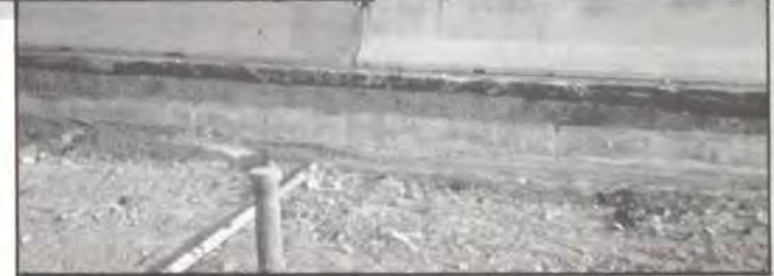
A view along the roadway reconstruction showing depth of cut, ELASTIZELL EF , aggregate base, asphalt road surface, and temporary traffic barriers.
