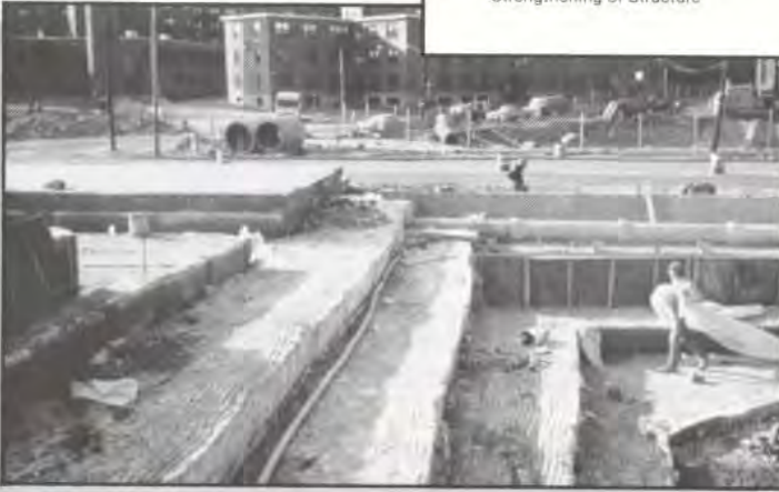
The 2 foot lifts of Class II ELASTIZELL EF were designed to reduce the load over the culvert structure.
