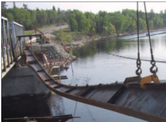
MTO recently used heat-straightening to correct an installation accident that occurred during the construction of the Frog Rapids Bridge.
