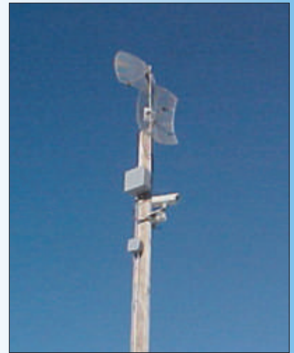
A monitoring camera with a microwave transmitter at the Kingston site.
